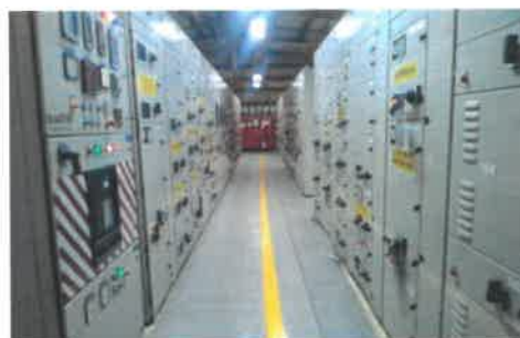
CS - 8 Electrical Sub Station
