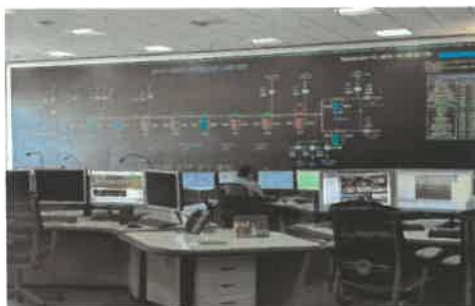
Pipeline Operation Centre - Control Room
