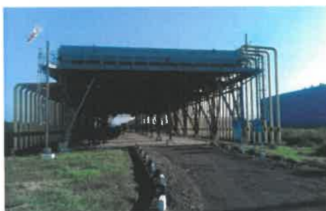
CS - 8 Gas After Cooler
